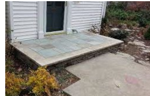
Private residence – single step with no handrails
